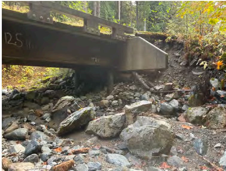
Eroded riprap at left bank
