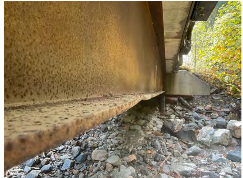
Minor damage noted along bottom flange
