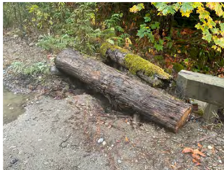
Downstream left bank erosion
