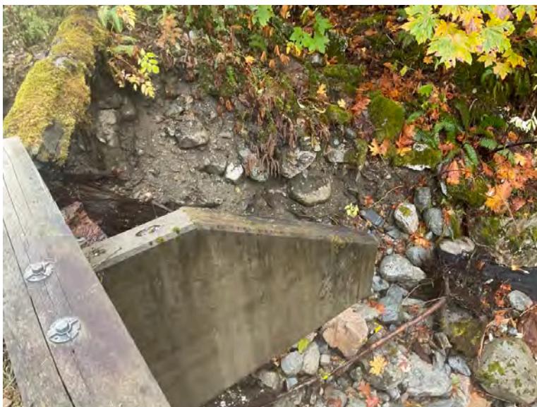
Downstream left bank erosion
